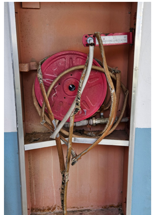
Figure 4.4 Damaged fire hose reel
