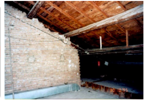
Figure 2.9 Incomplete fire barrier
