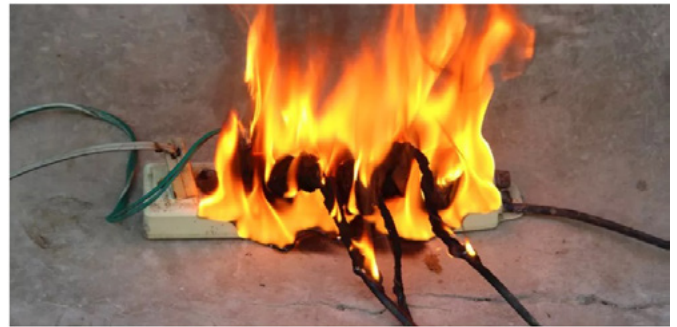
Figure 1.3 Fire involving overloaded electrical outlet / connections
