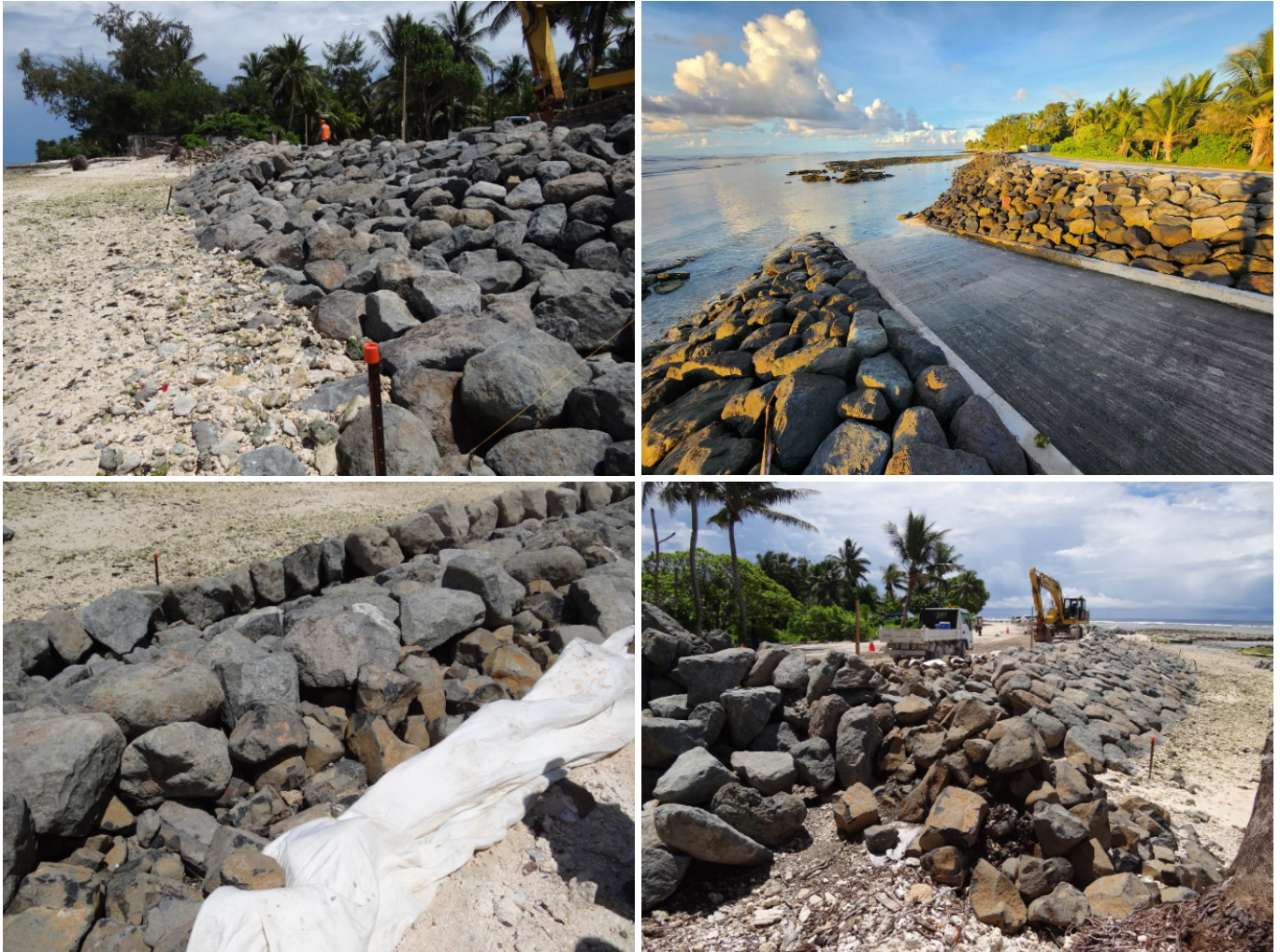
Construction of a Revetment. These photos show various stages in the construction of a coastal revetment in Temaiku, South Tarawa, with the bottom-right photo showing the revetment after completion. Source: The authors
