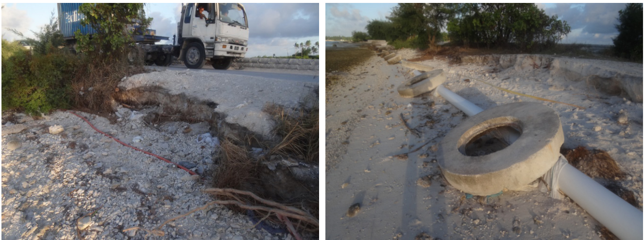
Erosion's dangerous effects. Coastal erosion is undermining roads (left) and utility infrastructure (right) in South Tarawa, Kiribati. Photo: Tom Shand.
