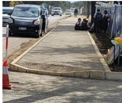
Access-for-All Facilities (Ramps for Wheelchair Users, etc.)
