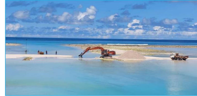
Clearing a boat channel in the Betio Bariki causeway of sand, Kiribati
