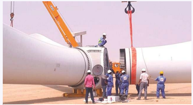
Source: Workers erecting a wind turbine at the Gul Ahmed Wind farm in Pakistan, Private Infrastructure Development Group (PIDG), 2015.
