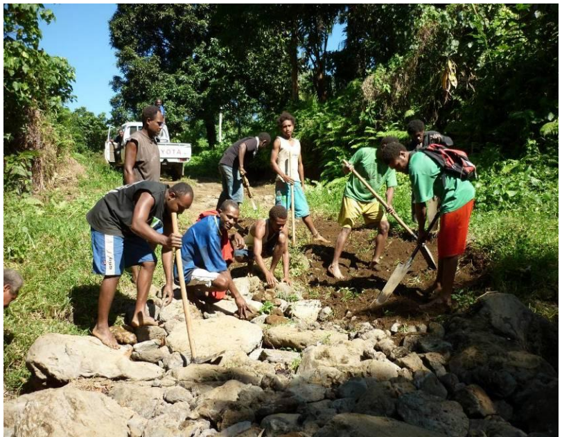
Lolovinue Villages in South Ambae carrying out emergency repairs to a river crossing on South Road that becomes impassable in and after heavy rainfall over the island
